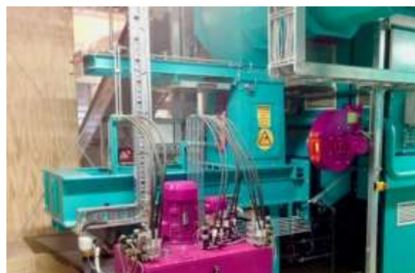
Fig. 20: Showing the ram feed. Note the gate valve above the day bin. And the hydraulic pack (pink).
