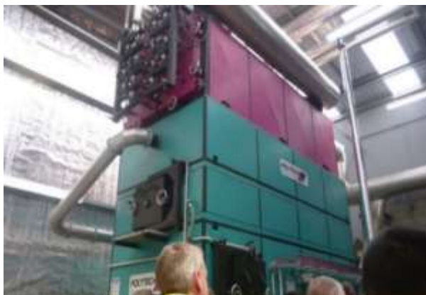
Fig. 5: The wood boiler at K&L Nurseries, 20 mins south of Christchurch
