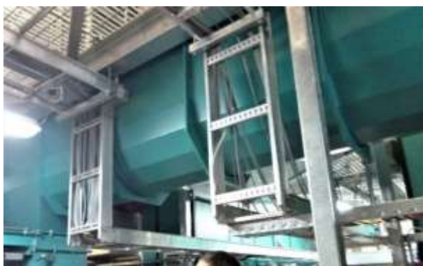
Fig. 19: Showing the dual-direction auger distributing fuel between the two boiler day bins
